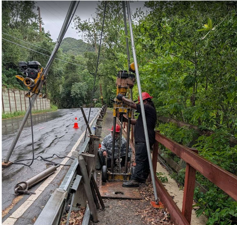
Image 2: View of Minuteman portable drill located between the guardrail and retaining wall railing.
